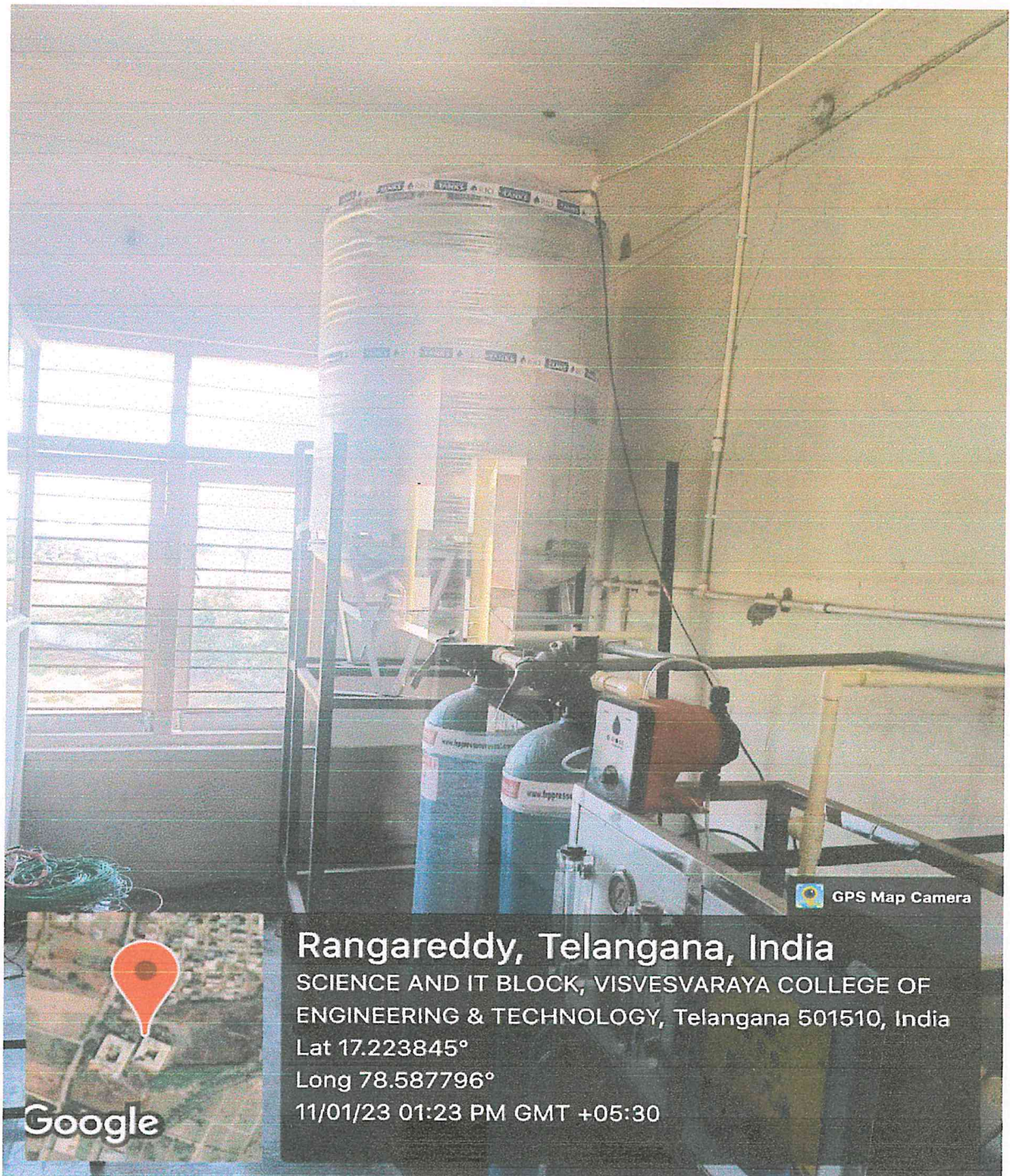
R-O Water plant in block B
