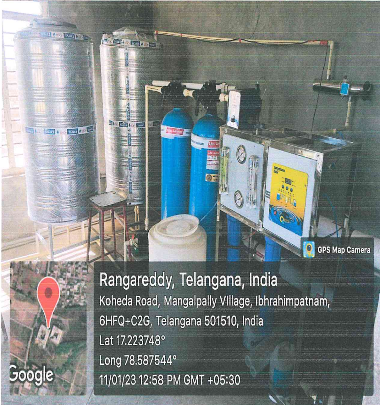
R-O Water Plant in main block
