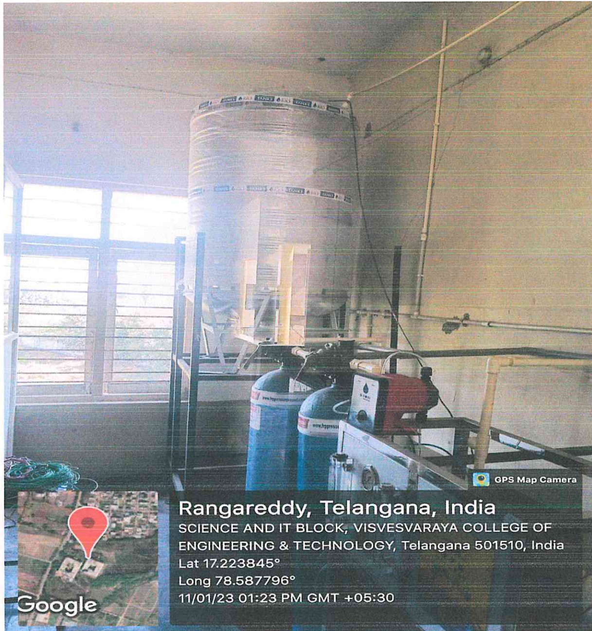
R-O Water plant in block B
