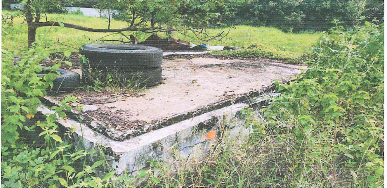
Rain harvesting pit Civil/Mech labs
