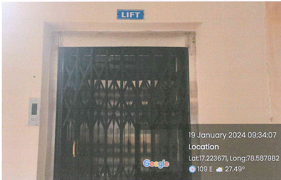
Lift at Block-B
